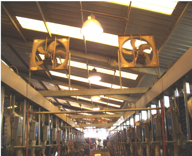
Figure 4-11. Example of panel fans for cooling milking parlor
