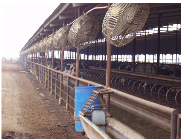
Figure 4-5. Circulator fans mounted under the eaves and taking advantage of prevailing winds.
