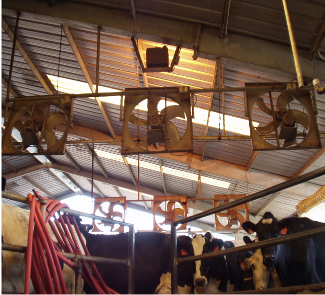
Figure 4-10. Example of panel fans for cooling holding area
