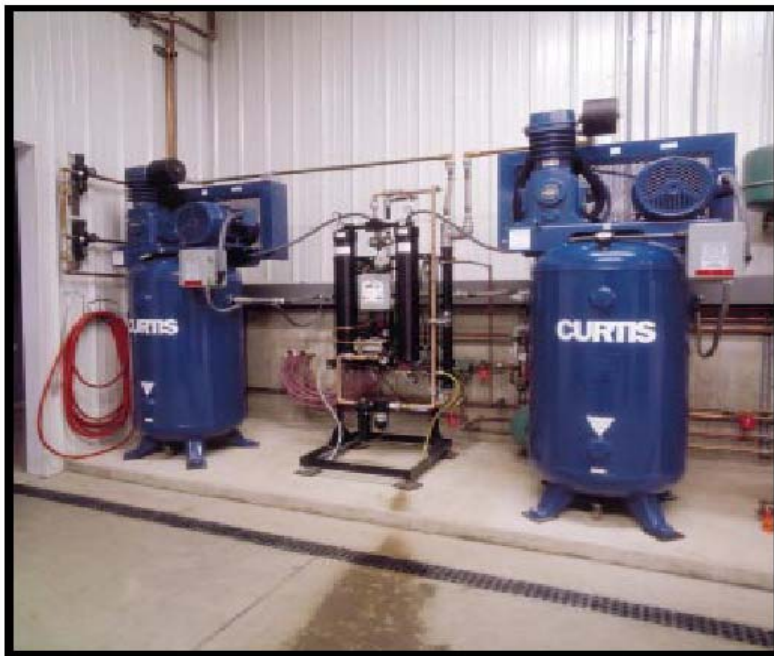
Figure 7-9. Compressed air system (Westfalia Surge)
