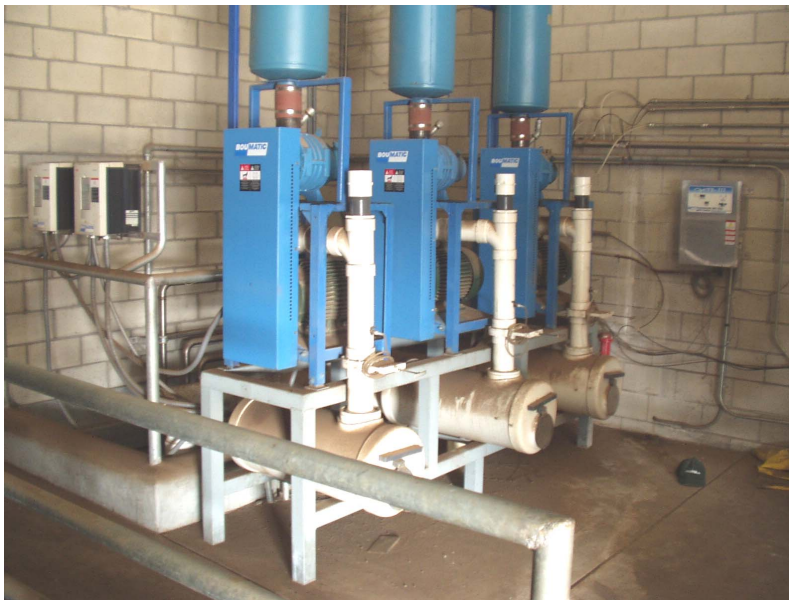
Figure 1-7. VFD vacuum pumps on California dairy
