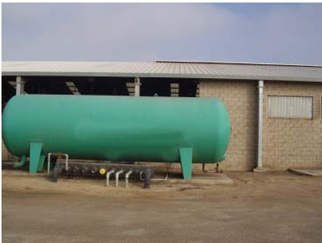
Figure 6-7. Pressure tank on California dairy
