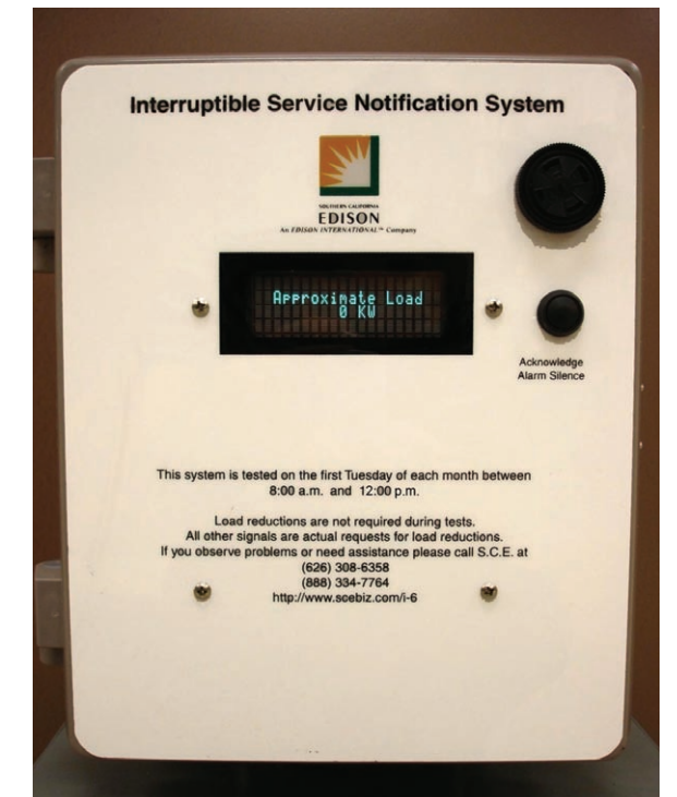
Figure 5: RTU Display Screen
